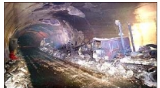
Aftermath of the Mont Blanc tunnel fire of March 1999 – the source of the fire was a truck carrying margarine and flour – the fire took 50 hours to completely extinguish
